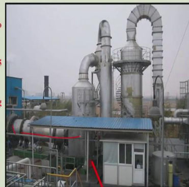
Rotary kiln incinerators in Henan province, China
