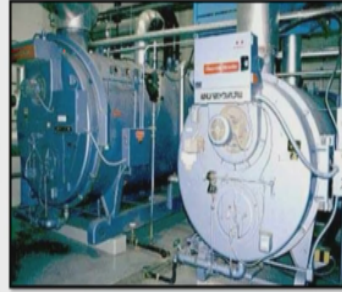
Boiler fuelled by landfill gas
