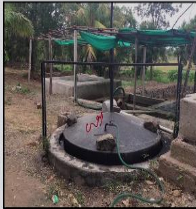
A community-level floating drum type biogas plant in India
