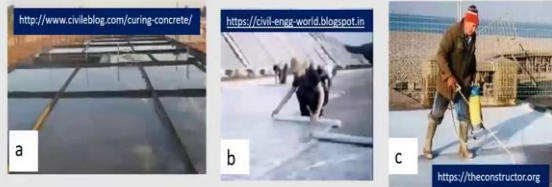
a) Wet curing, b) membrane curing, and, c) spraying of curing compound
