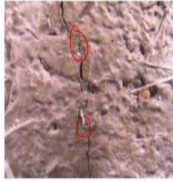
(25x25)mm Plastic shrinkage crack of hybrid steel - PP fibre Concrete
