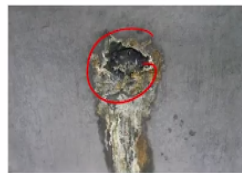
Air inlets blocked with ash; pungent smell and yellow deposit detected
