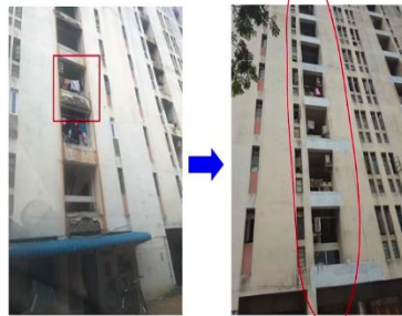
Patch repair without eliminating the moisture ingress and arresting corrosion can lead to repeated repairs in just a few years
