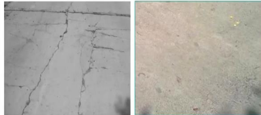
Significant cracking in plain concrete
