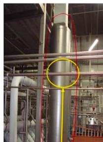
Column insulated against thermal cycling stresses
