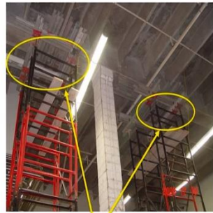
Design of shoring towers to support dead and live load during repair
