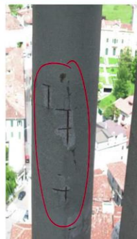
Spalling due to rebar corrosion
