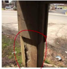
Spalling of concrete columns due to corrosion
