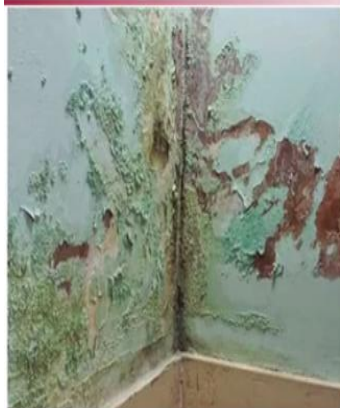
Blistering of paints at the corner of walls
