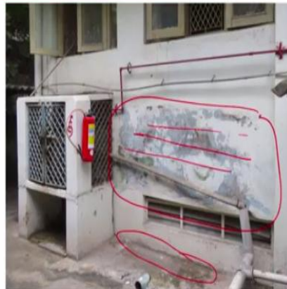
Dampness in wall due to capillary action
