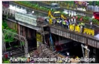
Andheri Pedestrian Bridge collapse
