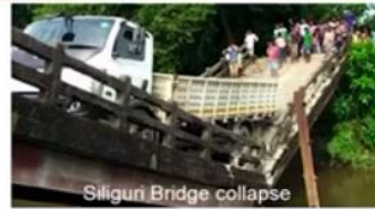
Siliguri Bridge collapse
