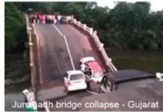
Junagadh bridge collapse - Gujarat
