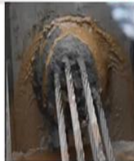
Signs of strand corrosion in a duct that was filled with water
