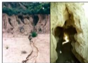
Fig. 5. Illustrates the rill process by showing soil surface erosion beneath the crest a) Rill formation with horizontal cracks b) Discontinuous rills with "hoop bridges" and c) Rill formation caused by soil heaving
