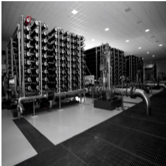
Typical reverse osmosis facility
