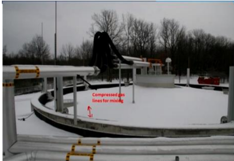
Anaerobic digester with floating cover. Flexible compressed gas lines allow for traverse of floating cover
