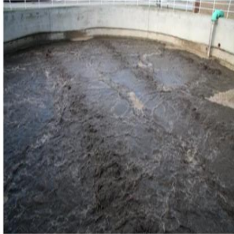
Aerobic digester under air. The solids concentration must be controlled. Concentrations above 4 percent will impede mixing and adequate dissolved oxygen levels. A concentration above 2 percent yields a smaller digester volume, a higher oxygen input per unit volume and increased levels of volatile solids destruction.
