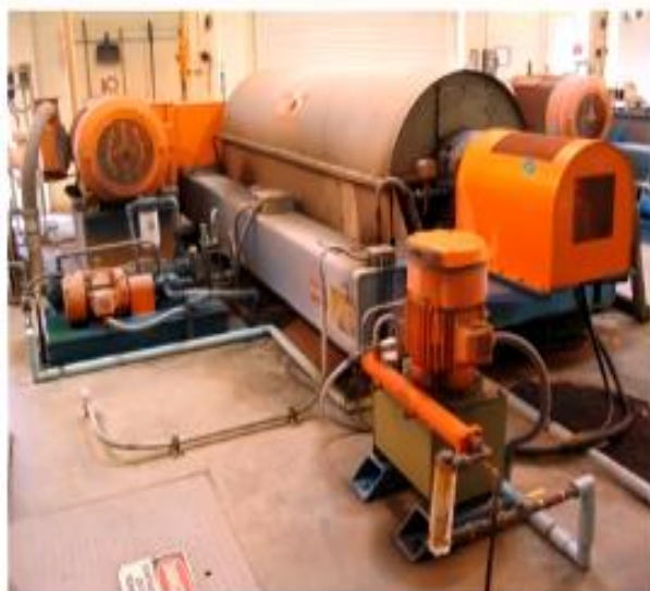
Sludge dewatering centrifuge
