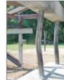
Buckled Steel Column
