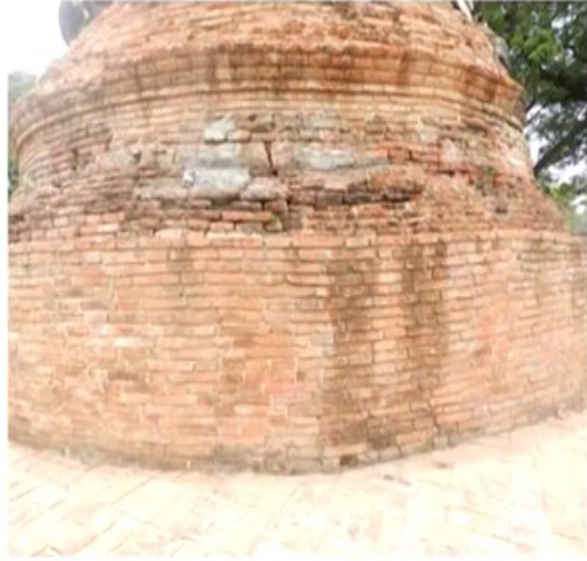
Reconstructed base - undulating brick layers not the best of workmanship
